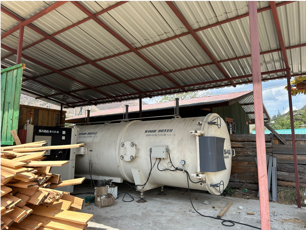
Figure 13 High Frequency Wood Dryer, Integrated Wood Processing Plant, NRDC, Ramtokto, Thimphu
